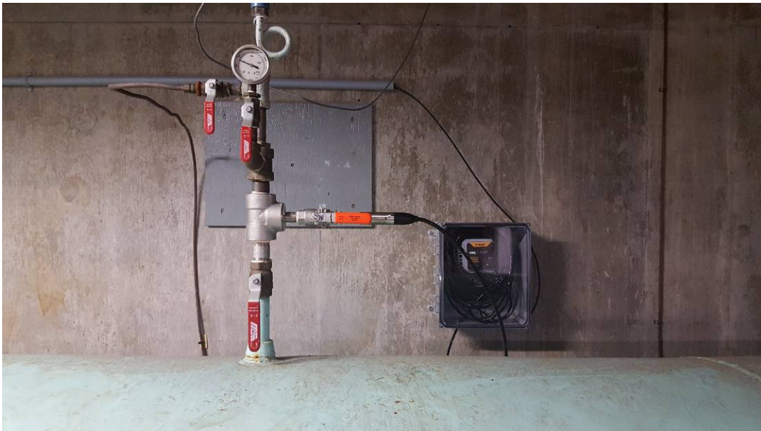
Figure 8: Pressure transient monitor installed in the primary transmission main.
