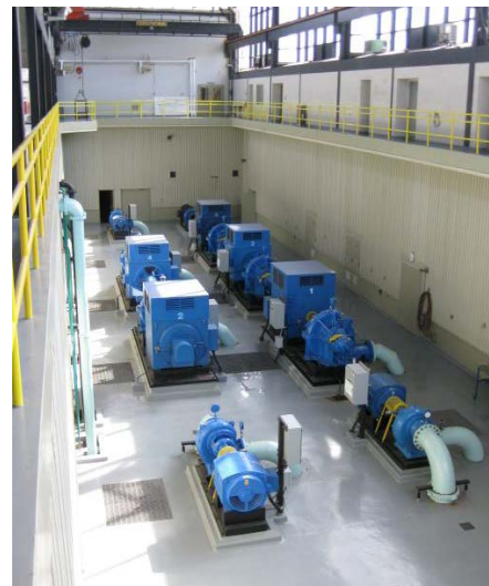
Figure 2: Pumps at the Lake Huron WTP
