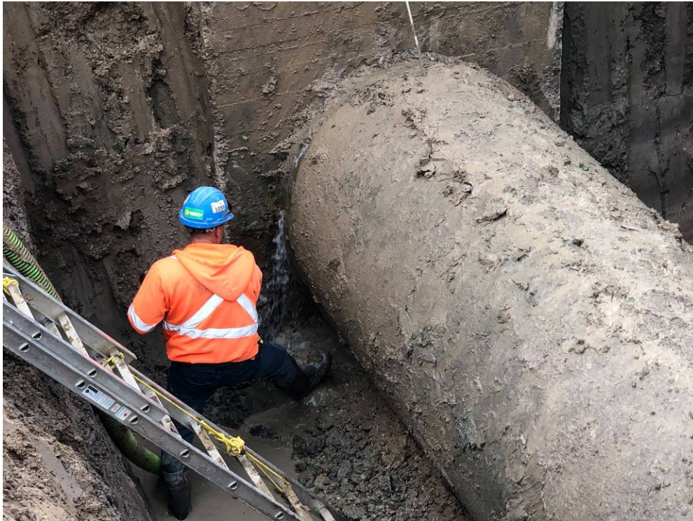
Figure 7a: After excavation to expose the pipeline and leaking joint, an inspection occurs.
